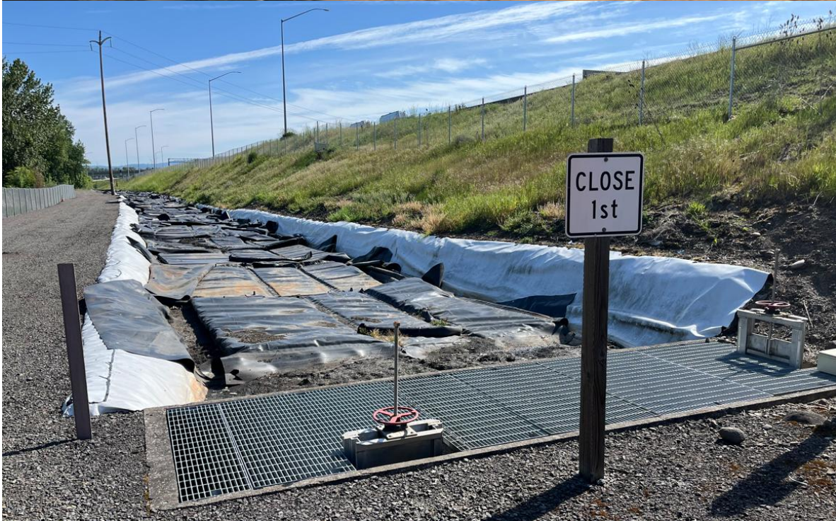
Figure 2: Oregon Department of Transportation (ODOT) modified water quality bioslope (DFI# D00652) photos from south side of facility looking north taken in 2013 during construction showing perforated pipes and media (top) and in 2025 showing floating rubber cover (bottom).
